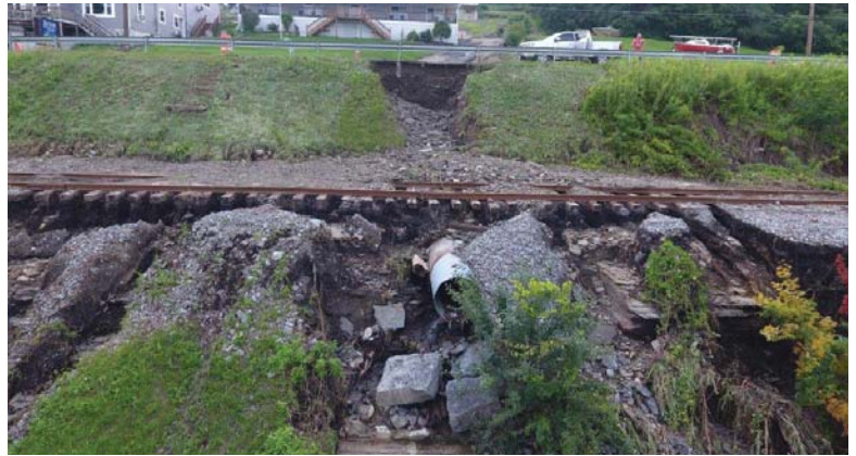
Culvert Erosion, June 2015 photo credit: Schuyler County Emergency Management
