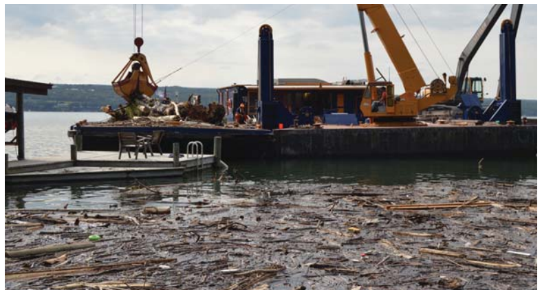
Clean up after August 2018 Flash Flooding along Seneca Lake shoreline photo credit: Schuyler County Emergency Management
